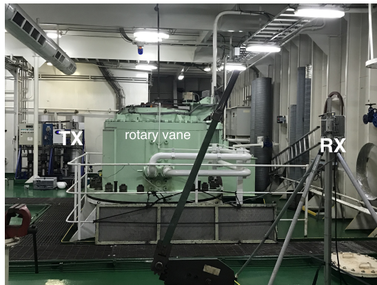
(c) Vane obstructing the Line-of-Sight path in steering gear room
