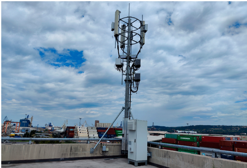
Figure 4. Logistic sector (port)—5G base station under test.
